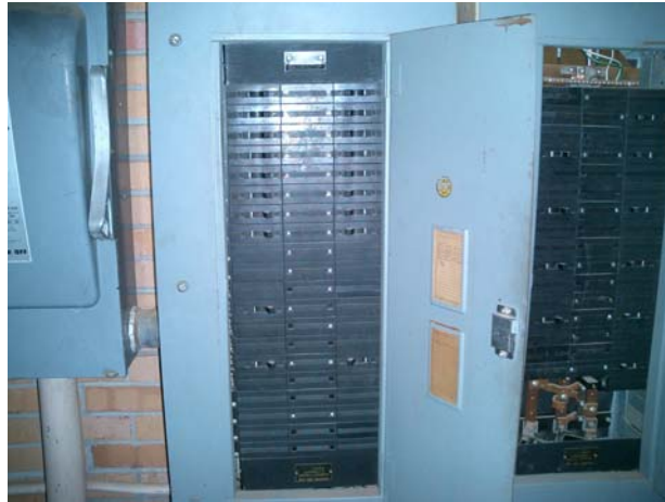
Figure 5: Alcorn State University Electrical Service Panel
